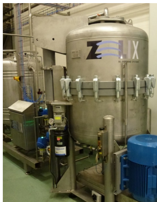
ZELIX 80-35 for wastewater from mayonnaise production - Picture right
